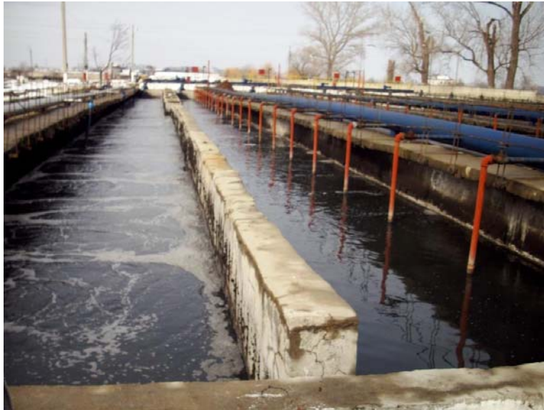
Fig. 8. Aeration in the biological reactor of Targoviste WWTP
