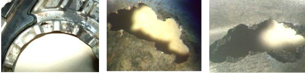
Figure 8. Corrosion in the crevice in the area of the circular cutout in the plate mark 4
