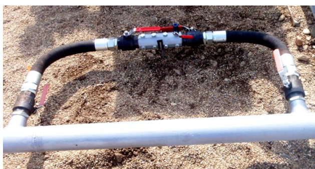
Fig. 1. The biofilm sampling device, installed as a by-pass of the injection water pipeline
